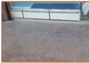
Fig 4.shows the variation of the finishing materials in some areas of the sidewalk, as well as the asymmetry in the sidewalk level. Source (Researcher)
