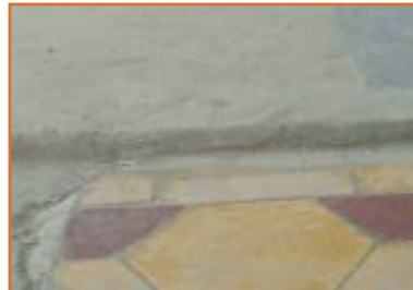
Fig (5)shows the variation of the finishing materials in some areas of the sidewalk, as well as the asymmetry in the sidewalk level. Source (Researcher)
