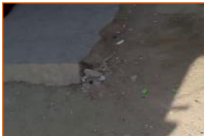
Fig(7) and Fig(8) show a discrepancy in the sidewalk level. Source (Researcher)
