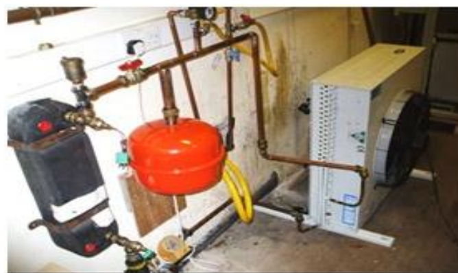
Fig. 3 Shows the connections of the heat exchanger, water pump, heat rejection fan and expansion valve.
