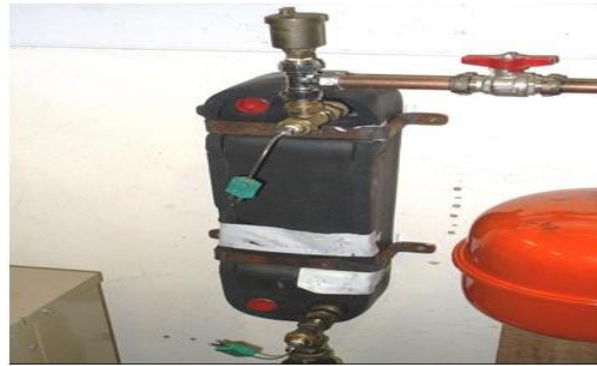
Fig. 2 Shows the heat exchanger.
