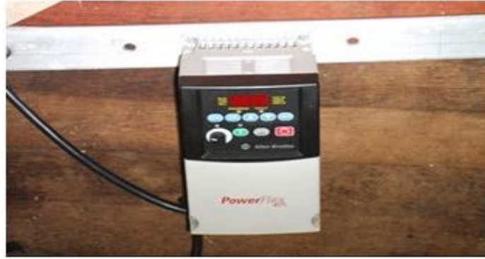
Fig. 5 Shows the power supply to heat injection fan.
